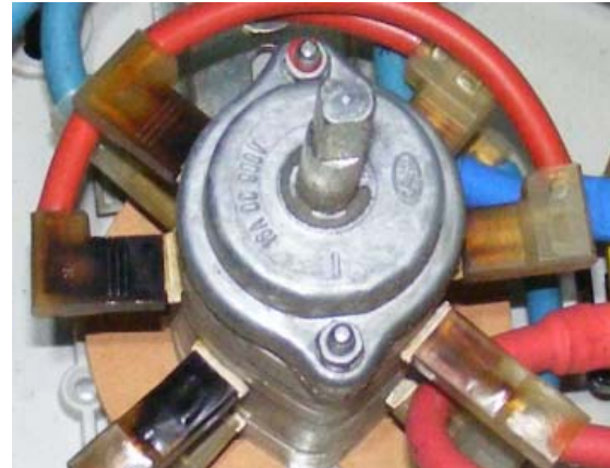
Figure 11: DC switch with charred terminals after six years of operation. This damage can be easily detected even by lay persons, if the contacts are visible.
