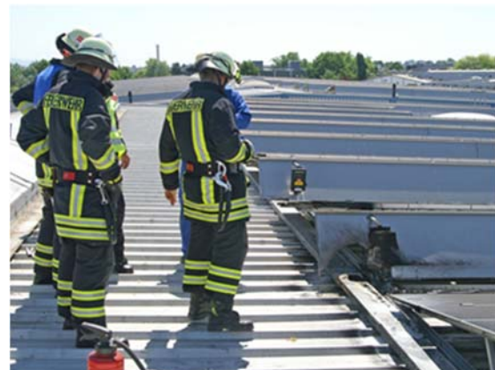
Figure 12: An array junction box had been destroyed by a fire. The j-boxes were fully exposed to sunlight and weathering. We assume that this exposure has contributed to contact degradation (photo: Freiwillige Feuerwehr (fire department) Bühl).
