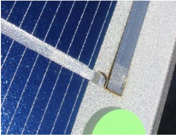
Figure 19: Close-up view of poor soldering. Without thermal imaging camera it is very hard to detect.
