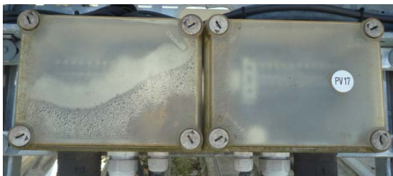
Figure 7: “Watertight” IP 65 array junction boxes after 15 years operation; the left one shows water droplets from condensed vapor.
